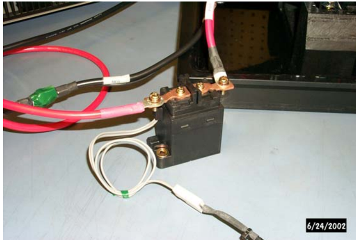
Figure 12: Installing the Load Relay
